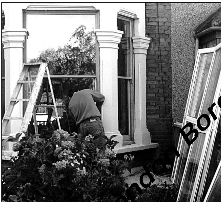
Unauthorised modern windows replaced by timber ones following legal action by the Council
