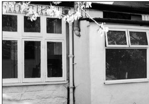
(Above) Original Loggias should be retained. The infilling by extensions, as here, is not acceptable.
